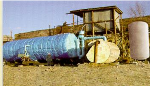
Figure 14. Biogas plant in Bartsrashen, Armenia (bioreactor 52m 2 )
