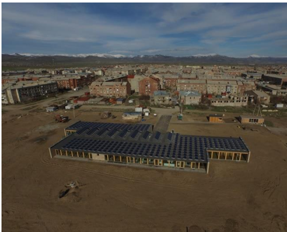
Figure 9. 95kWp PV station in Armenia was installed in Gyumri in 2014 by Caritas Armenia NGO
