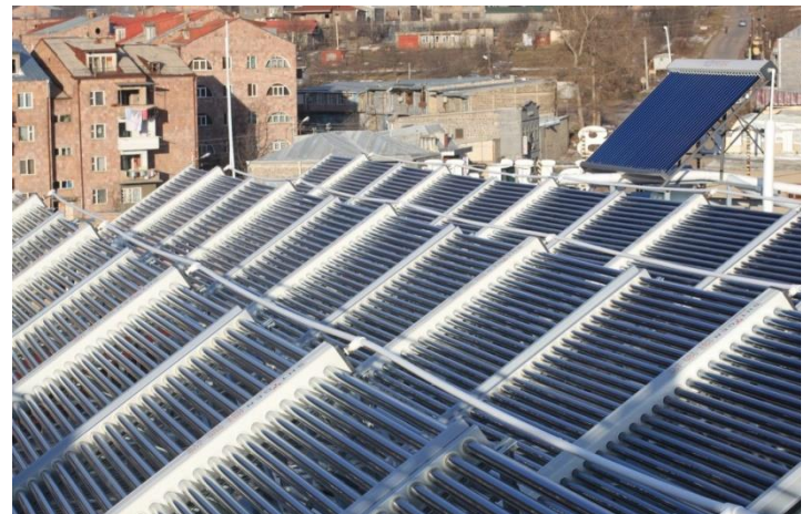
Figure 10. Solar water heaters at the roof of Hotel Diana in t. Goris installed by Shtigen Co.
