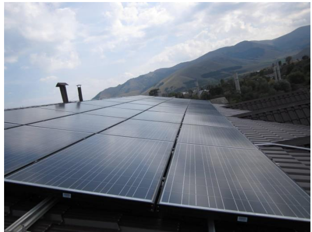
Figure 8. Grid-connected 17 kW Solar PV station at the roof of YMCA/Spitak building (2015)
