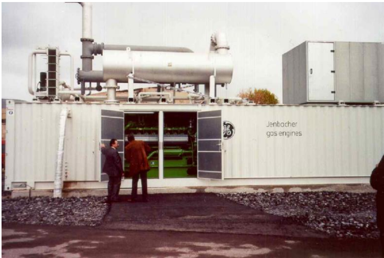
Figure 16. Jenbacher gas reciprocal engine with generator installed in container at LBP
